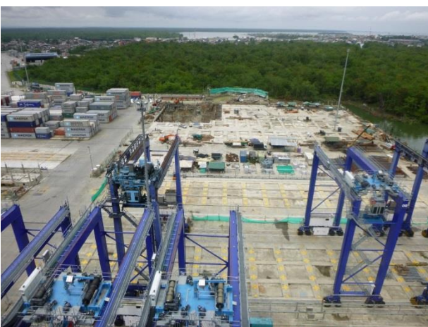
Caption: Construction site in Colombia: construction works for the extension of the terminal was happening parallel to the installation of the conductor rail systems and the modification of the RTGs
